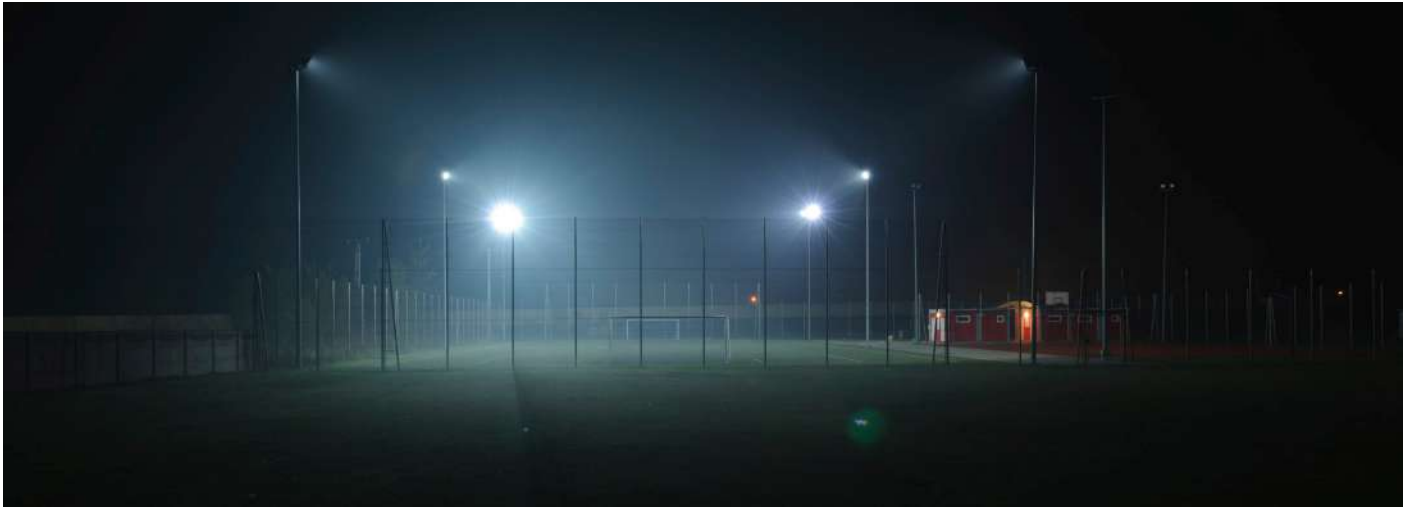
Thai Outdoor LED Floodlight Lighting Project ▼
