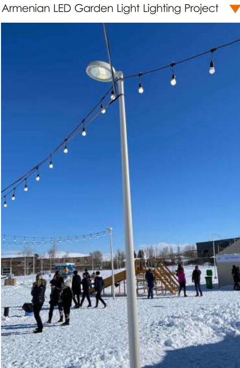
Amenian LED Garden Light Lighting Project ▼
