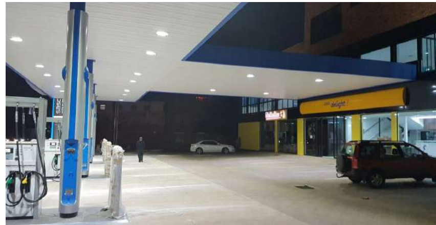
American LED Gas Station Lighting Project ▲
